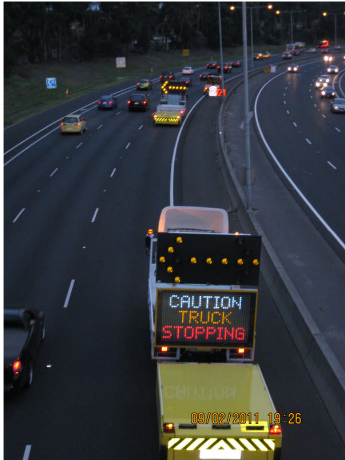
Eastern Freeway frequently moving works adjacent to fast lane. Advance warning TMA in foreground and shadow TMA in background protecting traffic management vehicle. The TMAs are protecting against both longitudinal and lateral errant vehicle entry into the work area.
