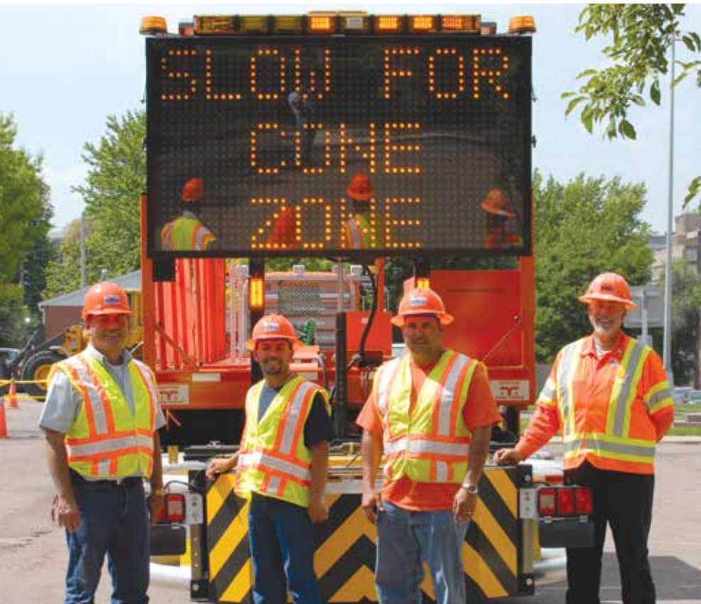
Above: Ken Maestas, supervisor, (on the left) and crew from the Colorado Dept of Transportation after setting up the first Mobile Barriers MBT-1 for CDOT's work zone safety event held at CDOT headquarters in Denver, Colorado, in June 2008.
