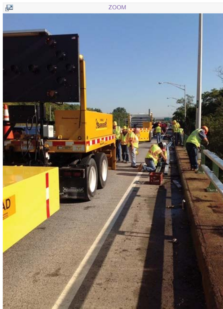
MB said that the effectiveness of its MBT-1 barrier was perfectly demonstrated in a recent project completed on the Korean Veterans Highway in Staten Island, New York
