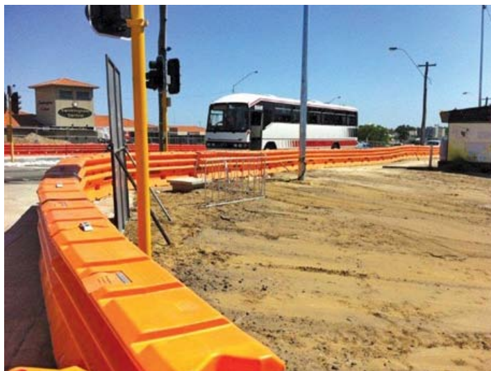
An application of Amorzone plastic barrier on a highway in Perth, Western Australia
